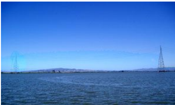
High Voltage Tower
